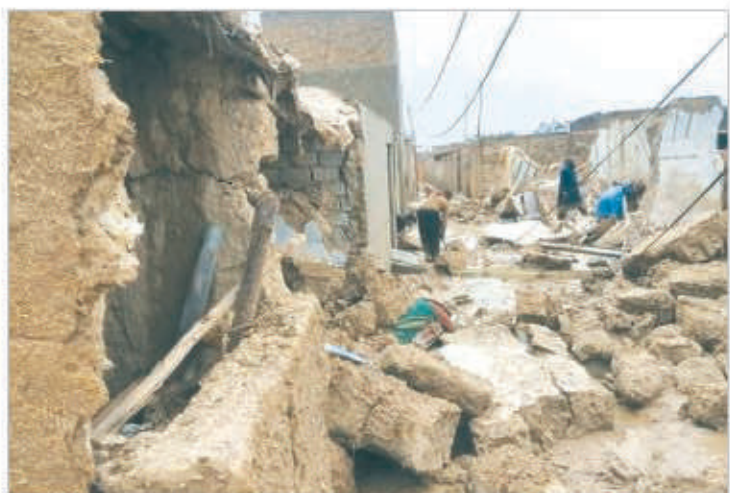
QUETTA: A view of damage house due to recent rain in Qila Saifullah.
