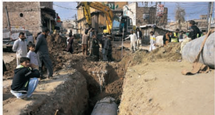
PESHAWAR: Labours busy in placing pipe during ongoing work progress at Afridi Ghadi Gulbahar no 4.
