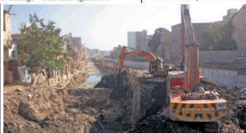
KARACHI: Workers are busy in cleaning Nulla with the help of heavy machinery at Pak colony area in Provincial Capital.
