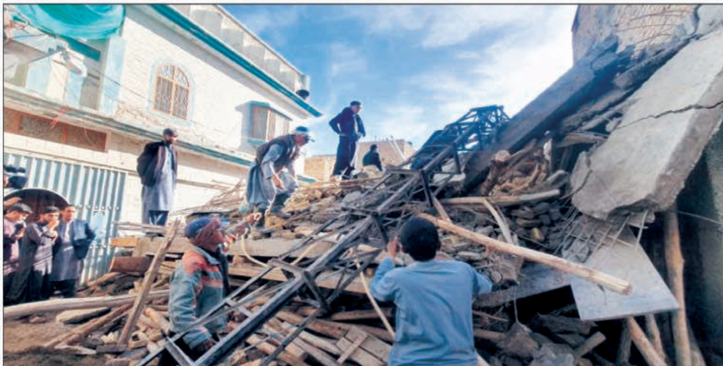
Rescue workers at the spot to retrieve the trapped laborers after the collapse of building on Stewart Road: Photo Manan Mandokhail
