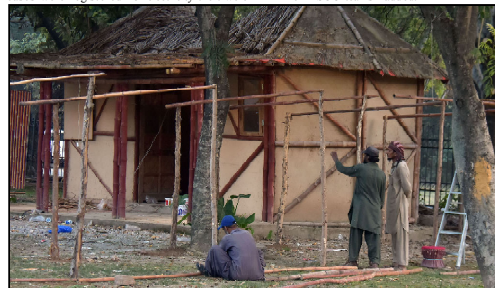
ISLAMABAD: Workers busy in preparing Sindh pavilion for up coming Lok Mela in Lok Virsa.
