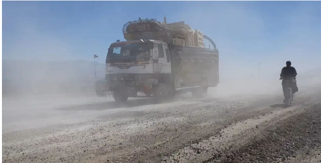
A view of the under construction Western Bypass in Quetta: Photo Daily Quetta Voice
