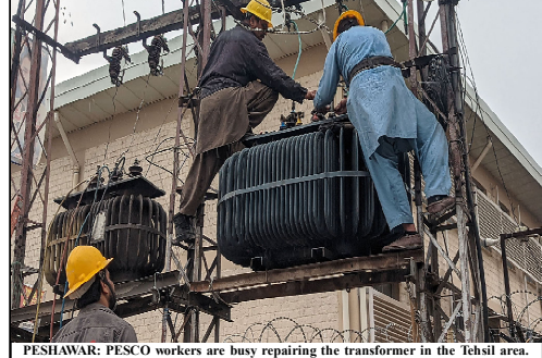
PESHAWAR: PESCO workers are busy repairing the transformer in the Ichsil area.
