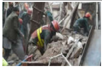
FRONT PAGE 14 children dead in Lahore tuition centre roof collapse... Page No 1
