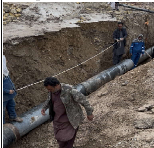
Technical team at the spot of the blast that damaged the gas pipe line:
